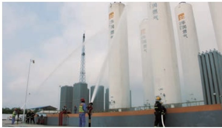
丹東華潤燃氣聯合消防部門開展應急演練 Joint emergency response drill of Dandong CR Gas and the fire department
